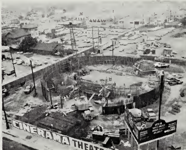
Getting ready for "It's A Mad, Mad, Mad, Mad World" premiere, new Pacific Cinerama Theatres is site of mad, mad, mad construction activity with only months to go before Nov. 7 deadline. Construction is proceeding on 24-hour basis, but nobody has doubts.
